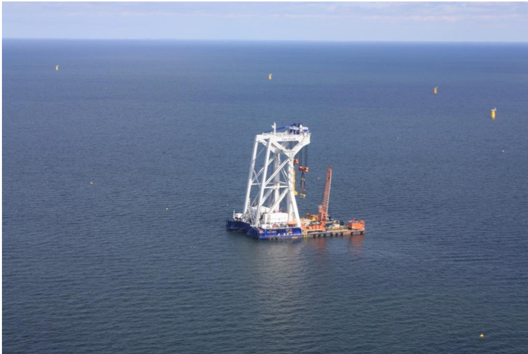
Figure 7. The pile-driving ship “Svanen” photographed during the aerial survey conducted in area MSI (03 July 2020) ©ITAW, Nadya Ramírez-Martínez.
